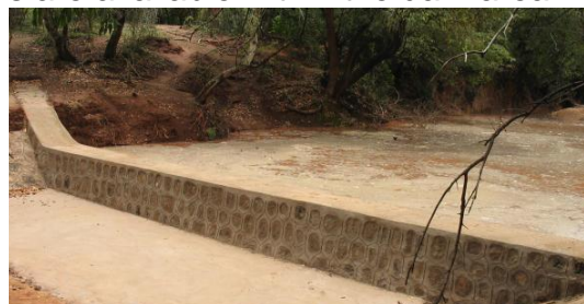
Figure 45: Stone-masonry sand dam after one runoff event in Borana, Ethiopia (Ethiopian Rainwater Harvesting association (ERHA), 2008).
